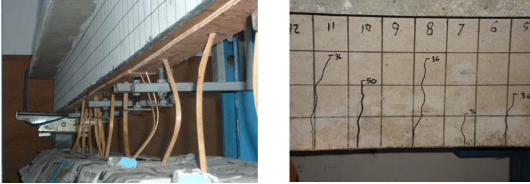
Figure 4. Installation of steel plate from underneath (left) and crack detail of beam at failure (right)
