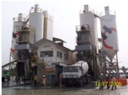
'Twin Batching Plant' Kuningan
